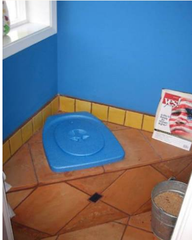
Figure 5: Composting toilet with Separrette diverting insert.
