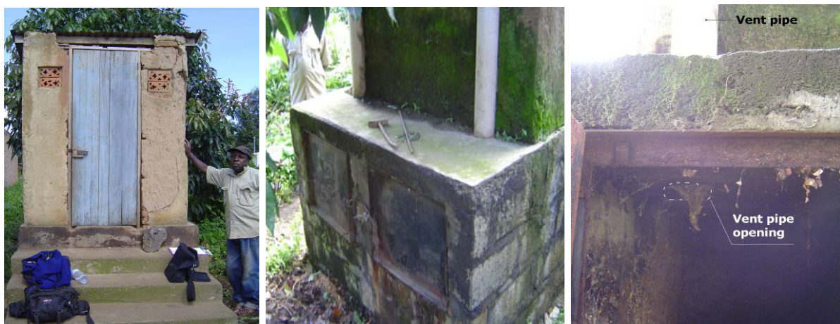
Figure 6.10.: (f.l.t.r.) Front view. Rear view (vertical doors; two outside vent pipes. Detail of the left chamber (vent pipe breakthrough)
