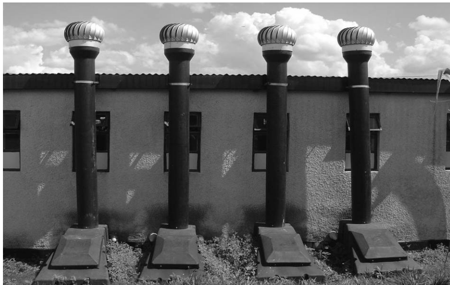
Figure 6.8.: Rear view of an Enviro Loo facility
