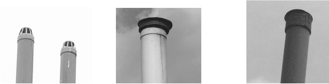
Figure 6.4.: Various rain shelters applied on vent pipes. Left picture represents a cover fitting in Bubaale, Kisoro Rd.; Middle image shows a combination of a cover fitting and a self constructed top piece; Right picture indicates a self construction without any space between the pipe and the shelter.
